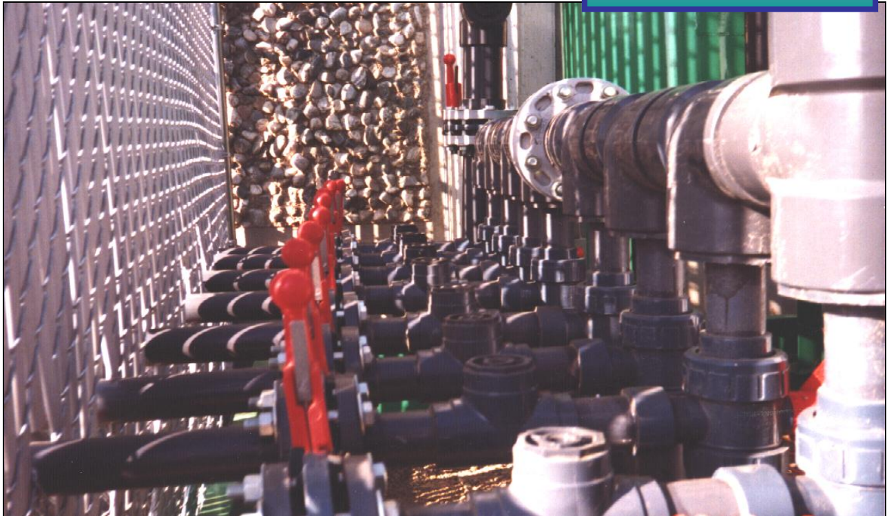
Manifold and valve system for soil vapor extraction and ground water treatment of VOCs.
