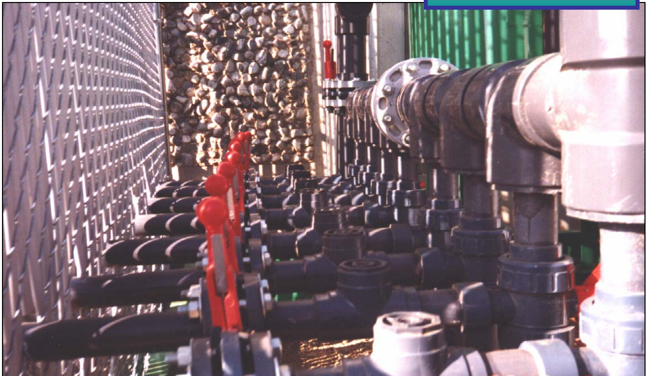
Manifold and valve system for soil vapor extraction and ground water treatment of VOCs.
