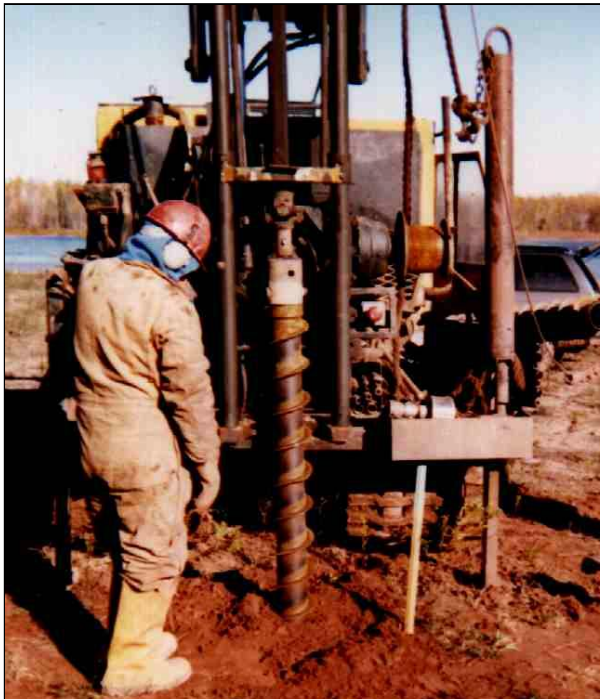
Focused, limited field investigation performed to characterize site conditions, quantify risks and estimate environmental expenditures.
